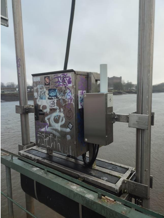
Figure 5: Installation of IW-NET component at existing shore power station (src: bremenports GmbH & Co. KG)
