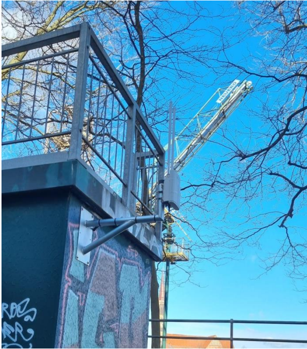
Figure 8: Gateway installed at bremenports facilities within Bremen (src: bremenports GmbH & Co. KG)
