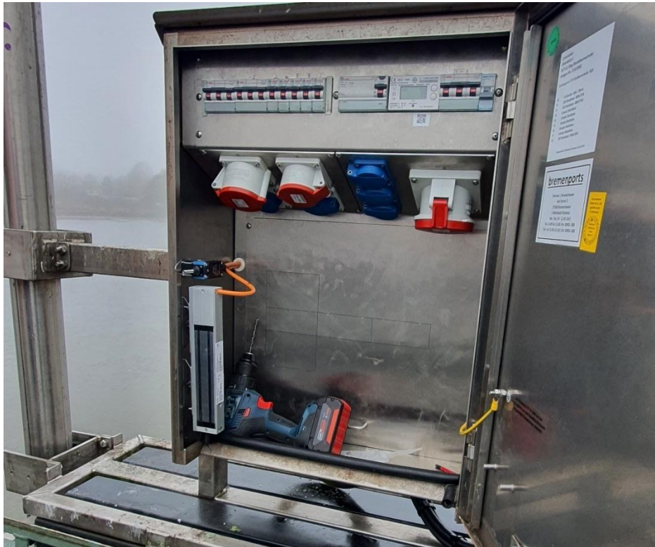
Figure 7: Magnetic opening mechanism within existing shore power station (src: bremenports GmbH & Co. KG)
